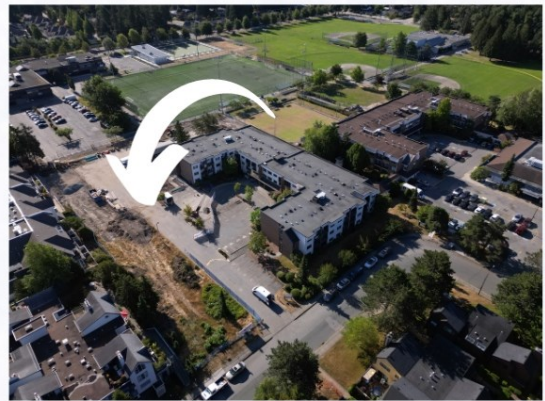
Arial view of construction for KinVillage Phase 1 Independent Living/Enhanced Day Program for Older Adults
